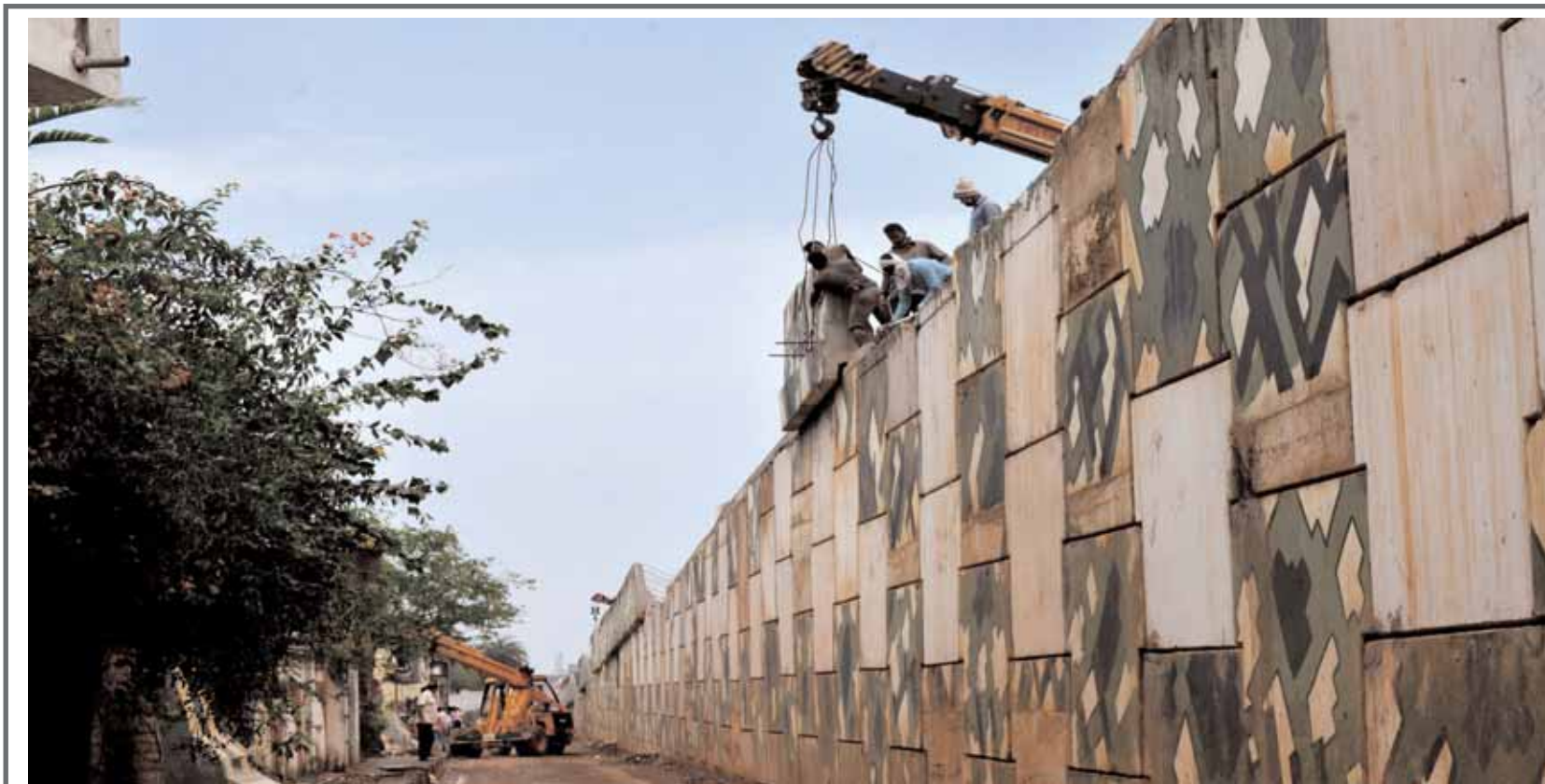
Heavy concrete blocks supporting the under construction Expressway near Shankar Nagar in Raipur fell on Monday. These were lifted safely. No casualties were reported. Pioneer Photo
