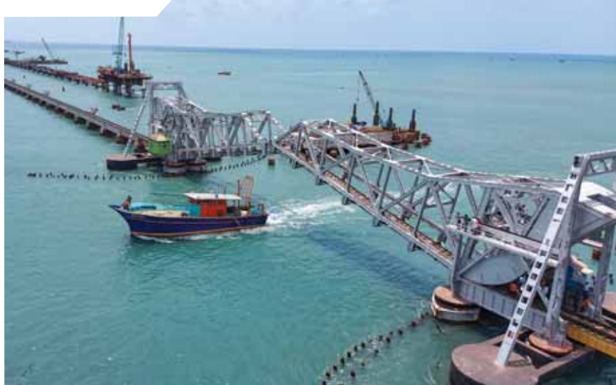
The Pamban railway bridge during its inspection by the railway officers, in Ramanathapuram
