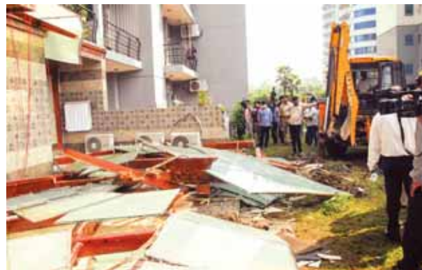
Residents gather as Noida authority carries out demolition of illegal construction at the Grand Omaxe society in Noida on Monday
