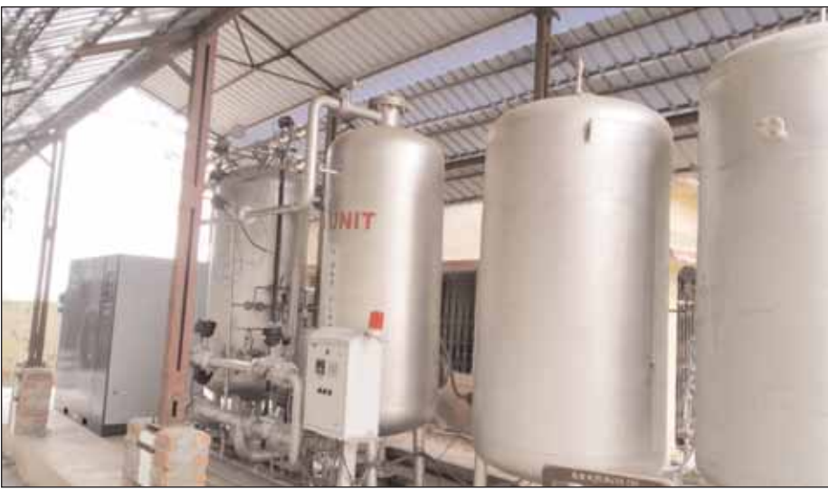
A view of Oxygen generation plant at Central Coalfields Limited (CCL) hospital in Ranchi on Tuesday. Pix by Vinay Murmu
