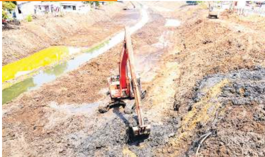
An excavator being used for the removal of silt from Bandar Canal at Tadigadapa, near Vijayawada, on Monday. Pic by Ch Vijaya Bhaskar
