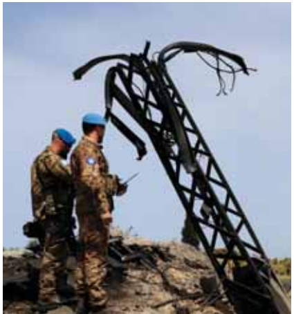
Italian UN peacekeeper soldiers inspect a small bridge that was destroyed by an Israeli airstrike, in Maaliya village, south Lebanon on Friday as Israel launched rare strikes in southern Lebanon early Friday.
