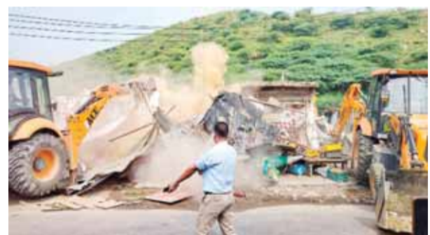
Illegal construction being bulldozed by the authorities during the third day of the demolition drive in violence-hit Nuh district on Saturday PTI
