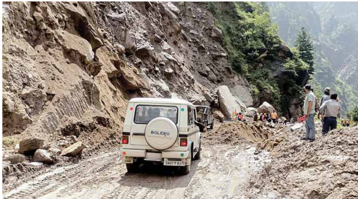
Restoration work underway at the Govindghat for the opening of the Badrinath national highway which was blocked due to landslides in Chamoli district on Tuesday. The Badrinath National Highway near Chhinka was blocked due to falling boulders from the hill on Friday morning. As a result of the highway closure, commuters, including pilgrims and tourists traveling to and from the famous Badrinath shrine have been stranded PTI
