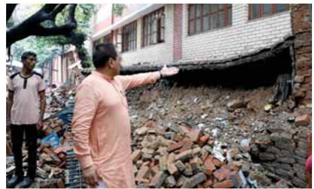
Delhi BJP president Virendra Sachdeva visits the site after a wall of a government school collapsed following rain at Garhi Jharia Maria Ranjan Dimri | Pioneer
