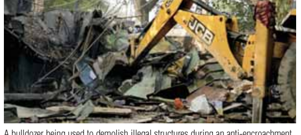
A bulldozer being used to demolish illegal structures during an anti-encroachment drive near Pragati Maidan, in New Delhi on Thursday
