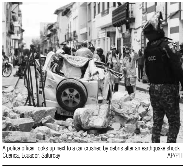
A police officer looks up next to a car crushed by debris after an earthquake shook Cuenca, Ecuador, Saturday. AP/PTI
