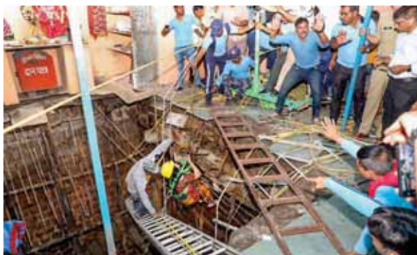
Rescue operations underway after the roof of a well collapsed at Beleshwar Mahadev Jhulelal, in Indore, on Thursday. At least 14 people got killed and several others are feared trapped, according to officials PTI
