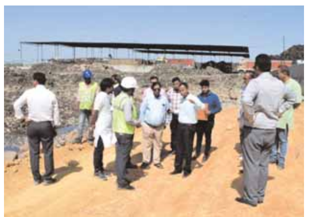
Commissioner visited the site and curtain wall. In view of the convenience of vehicular movement for the purpose make a temporary ramp with stones and marble.
