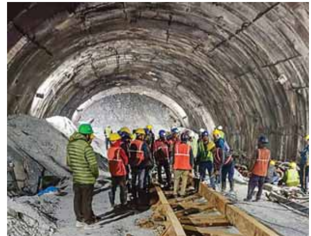
Rescue and relief operations underway after a portion of a tunnel under construction between Silkyara and Dandalgaon on the Brahmakhal-Yamunotri national highway collapsed, in Uttarkashi district, on Tuesday
