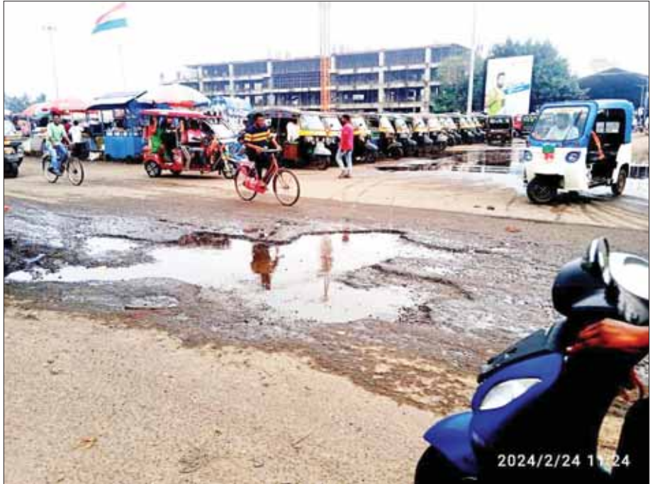
The authorities are unconcerned even though the road in front of the Puri railway station continues to remain in a dilapidated condition for months. Ranjan Ganguly
