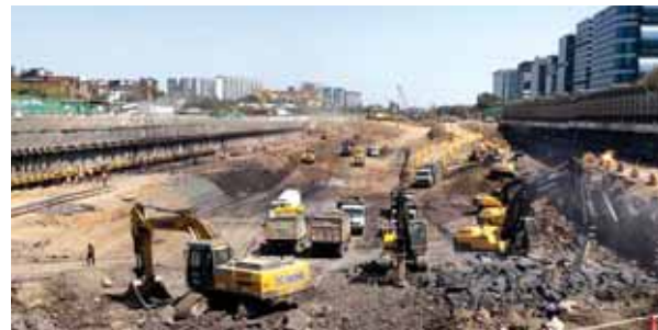
Construction work at the Bandra Kurla Complex Station, a key component of the Mumbai-Ahmedabad High-Speed Rail corridor. Photo by Deepak Kumar Jha
