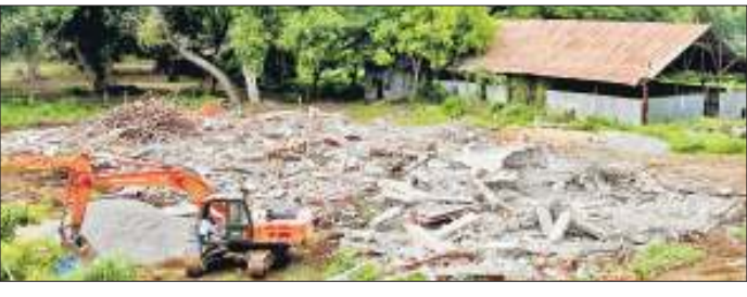
MMTC officials demolished the under-construction YSRCP Central Office at Sasetanagaram on Saturday. Pic by Ch Vijaya Bhaskar
