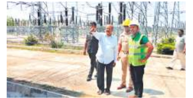
CMD of Souther DISCOM Musharraf Farooqui inspecting the damaged 220 KV transmission line at Miyapur sub-station
