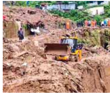
He said heavy rain was affecting rescue operations at the disaster site. The rain triggered landslides at several other places in the state and at least two persons have been "swept away", Shukla said.
