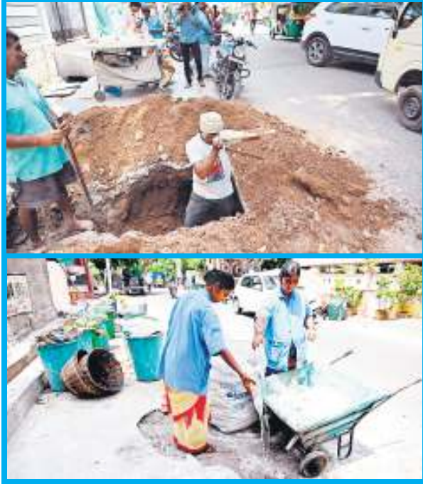
Municipal workers repair the drinking water pipelines at Patamatavari Street in Mogalrajapuram area of Vijayawada on Thursday. Pic by Ch Vijaya Bhaskar
