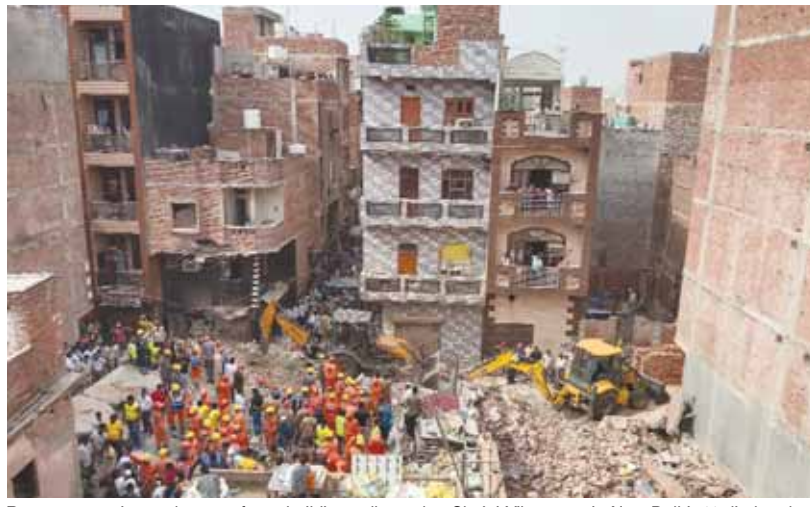
Rescue operation underway after a building collapsed at Shakti Vihar area in New Delhi. 11 died and several others are feared trapped after the four-storey building collapsed. RANJAN DIMRI/THE PIONEER
