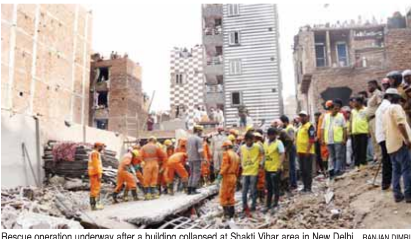
Rescue operation underway after a building collapsed at Shakti Vihar area in New Delhi, ranjan dimri
