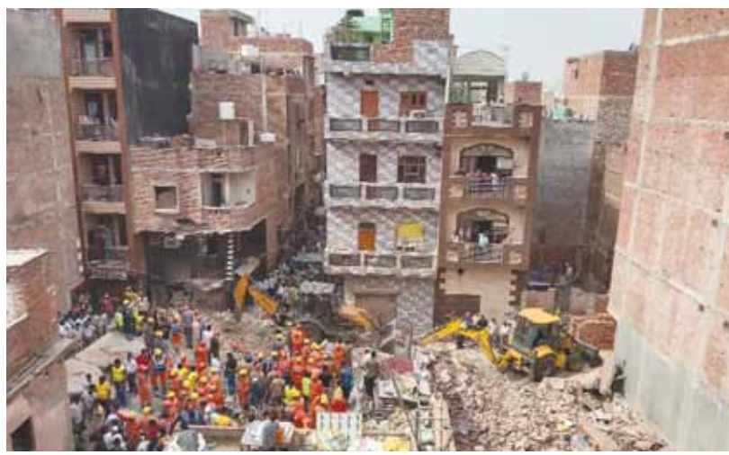
Rescue operation underway after a building collapsed at Shakti Vihar area in New Delhi. 11 died and several others are feared trapped after the four-storey building collapsed. RANJAN DIMRI/THE PIONEER
