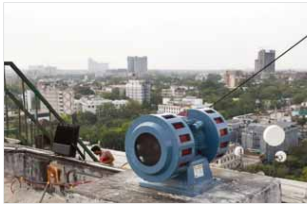
An air raid siren installed atop the multistorey PWD building at ITO
