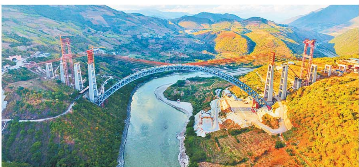
Aerial photo taken on Dec. 9, 2018 shows the railway arch bridge across the Nujiang River in southwest China's Yunnan Province. With a grand arch bridge erected on Monday morning, Chinese constructors have built the longest-spanning railway arch bridge with a single span of 490 meters. The bridge is a key project of the 220-km-long Dali-Ruili railway which is a key section of the China-Myanmar international railway corridor linking Kunming, the provincial capital of Yunnan, with Yangon of Myanmar
